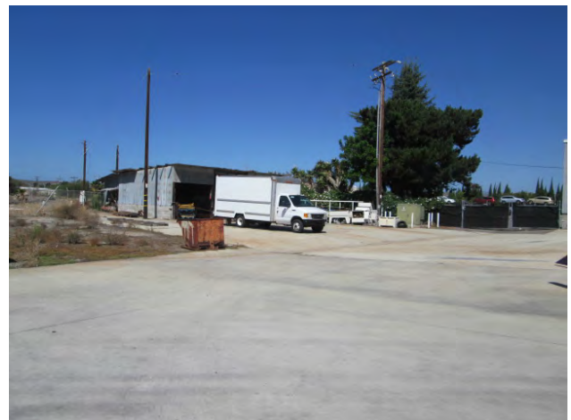
18. Shed and pad mounted transformer located west of the main warehouse.
