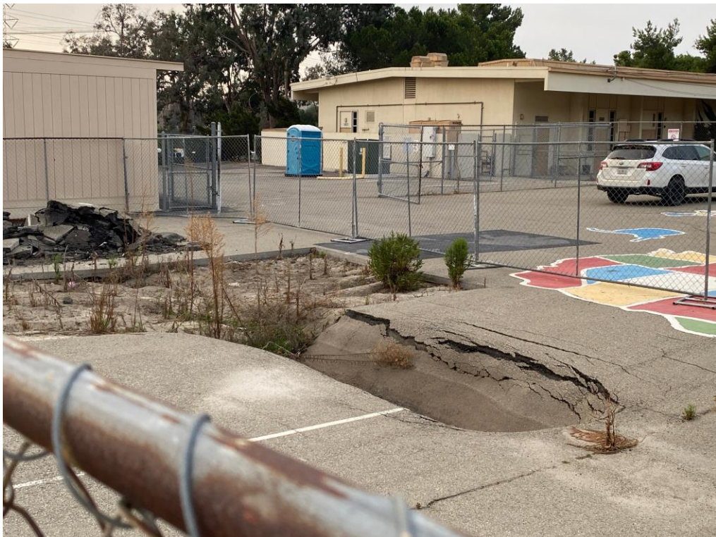
26. View southeast, of surficial damage from storm drain.
