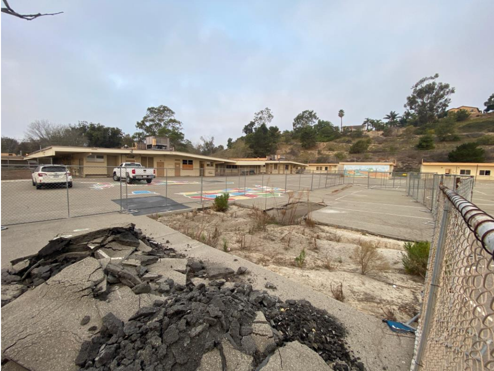
25. View southwest, of surficial damage from storm drain.
