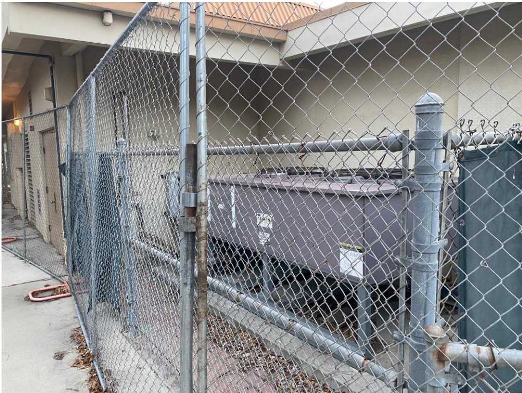
8. View north of typical Air-Conditioning Unit.
